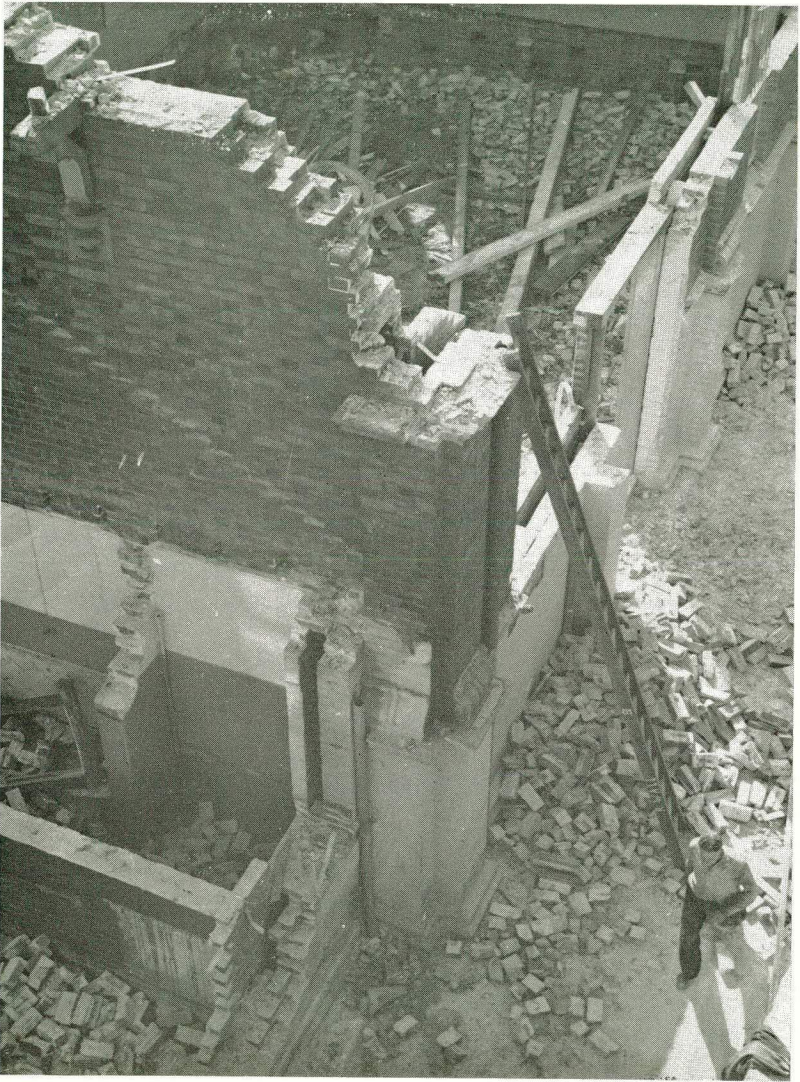
The Demolition of the 'Prep.' building to make way for the extended Science Building
